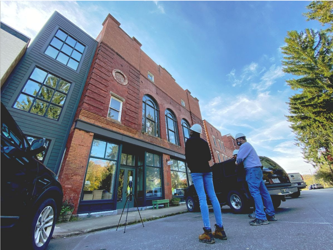
The Mills Group onsite last week, scanning the exterior of Cottrill's Opera House (note the Leica scanning unit, on a tripod near the sidewalk).
